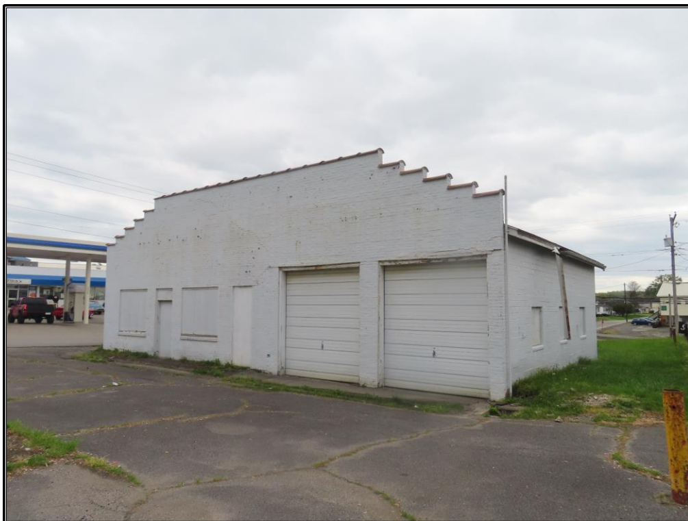
Figure A-18. BD 84: Façade and northwest elevations of the building, looking south.
