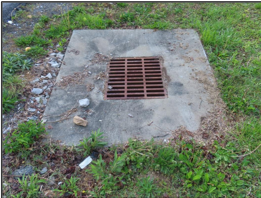
Figure A-22. CRA B: Pipe culvert in concrete basin north-northwest of KY 168/Bellefonte Road intersection, looking south-southeast.
