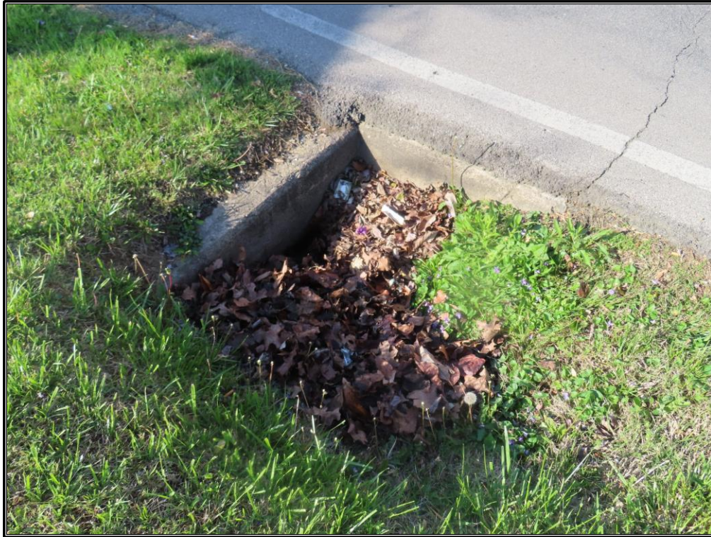
Figure A-21. CRA A: Pipe culvert at KY 168/Woodland Avenue intersection, looking south-southwest.
